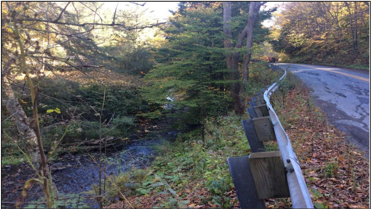
Figure 1-3: Unstable Guiderail and Road Stress Fractures on North bound side of SR 1005
