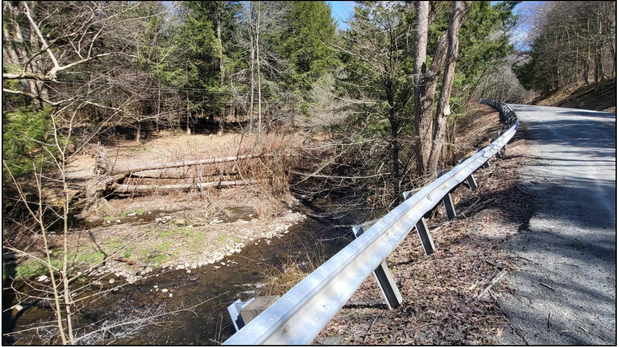
Figure 1-2: Gravel Bar in Starrucca Creek and Unstable Guiderail Along North side of SR 1005
